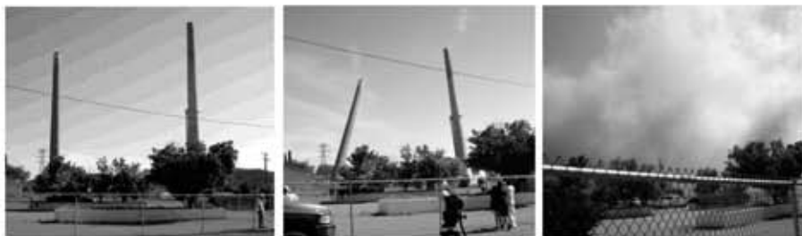
Photos of Hurley smelter stack demolition taken from Chino Blvd. and Romero St., southwest of the stacks.
